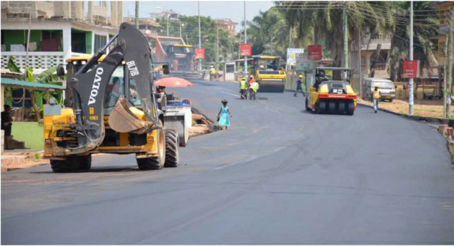
EMERGENCY ASPHALTIC OVERLAY ON SELECTED ARTERIAL AND COLLECTOR ROADS IN TAKORADI METROPOLIS (100 KM)
